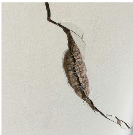
Close up of crack in the entrance lobby showing evidence of past repair
