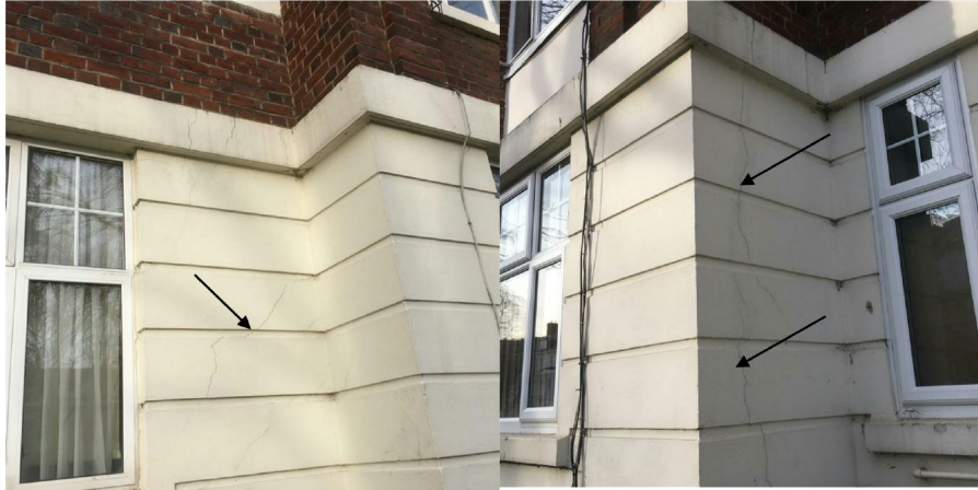
Cracks to front elevation
