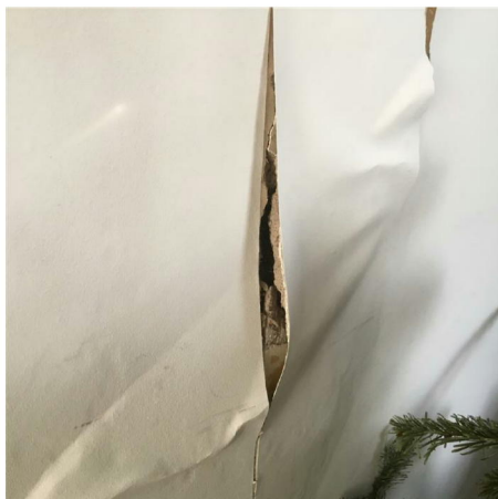
Crack in Flat 28 living Room
