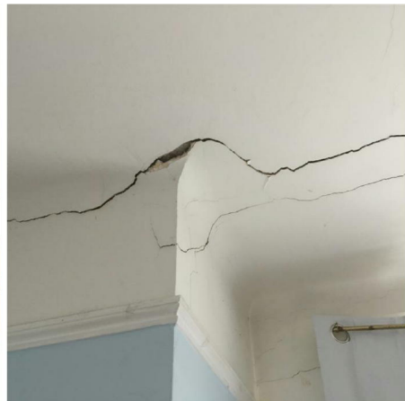
Cracking in Flat 2
