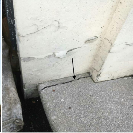
Damage to front steps at main entrance
