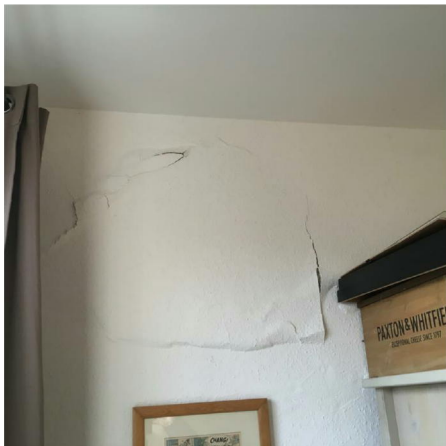
Cracking in Flat 28 Right hand end bedroom
