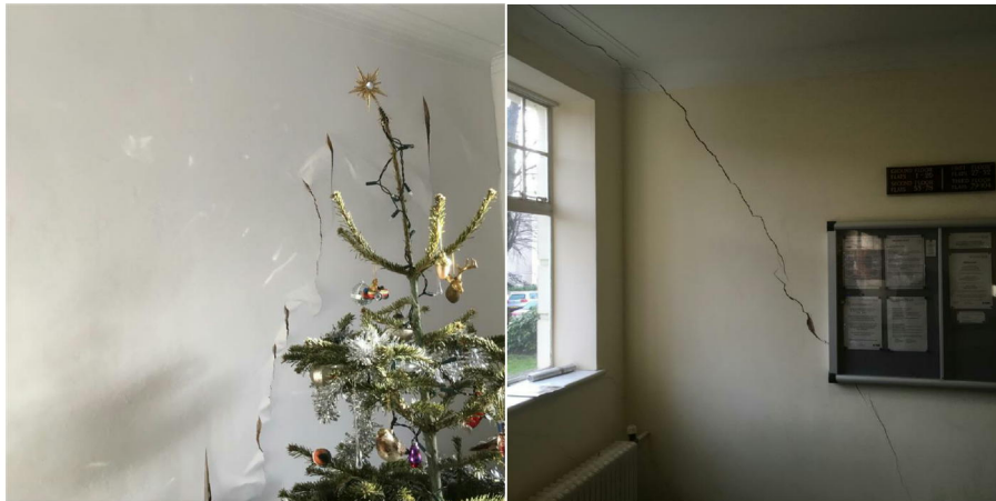
Crack in Flat 28 Living Room
