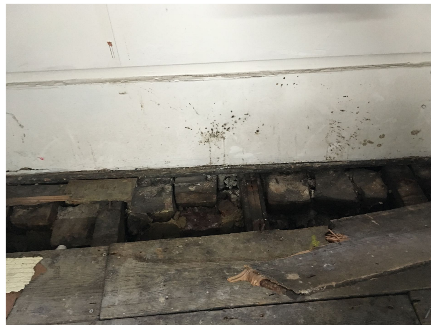
IMG_6640 Damage to floor boards caused by failure and detachment of front elevation
