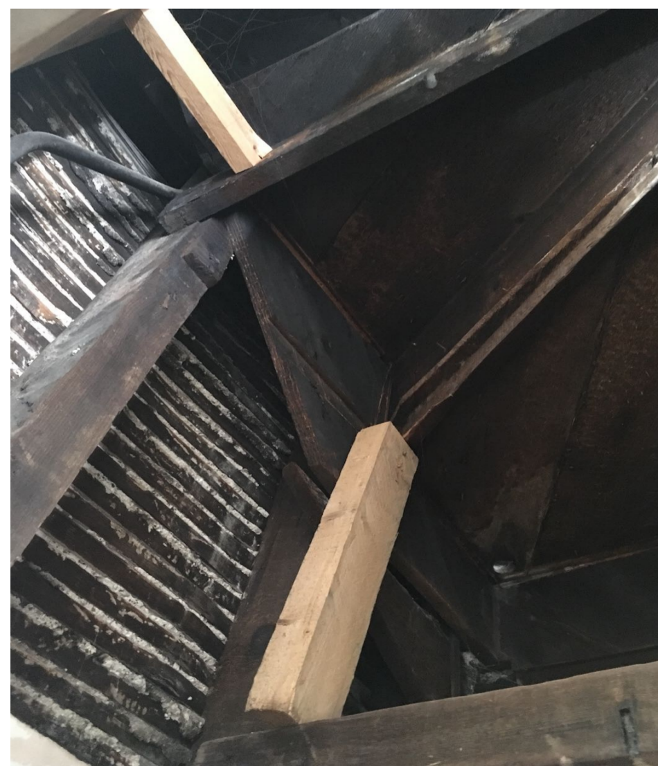
IMG_6975 Second Floor Fire Damaged to TOR204-Stair Soffit
