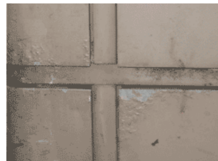
Because it is only a coating, painted aluminium can suffer surface failure over time
