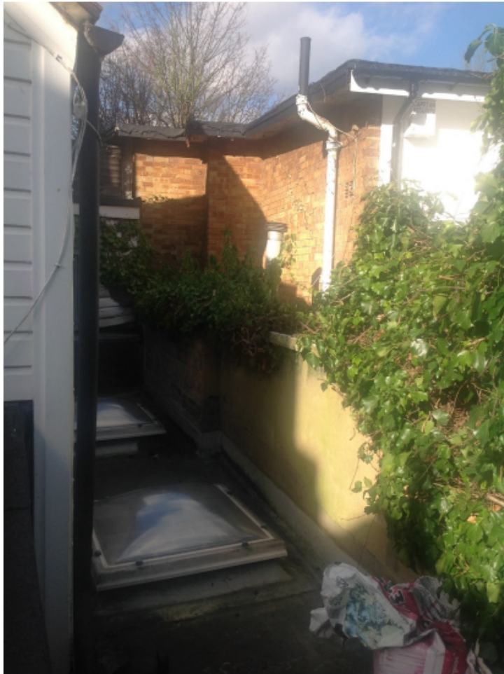
15. Flank wall of No. 2 Upper Park Road adjoining rear of 150a Haverstock Hill
