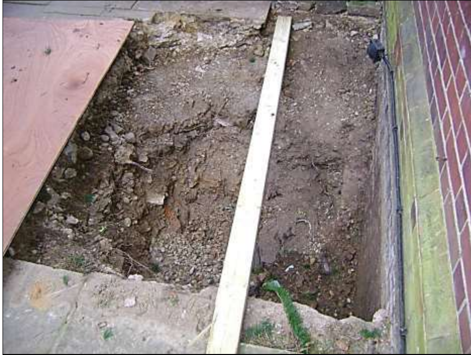
Photograph 3 – Looking into the trial pit dug on one corner of the proposed extension. Only a few minor fibrous roots have extended below the hard-core base of the stone patio.
