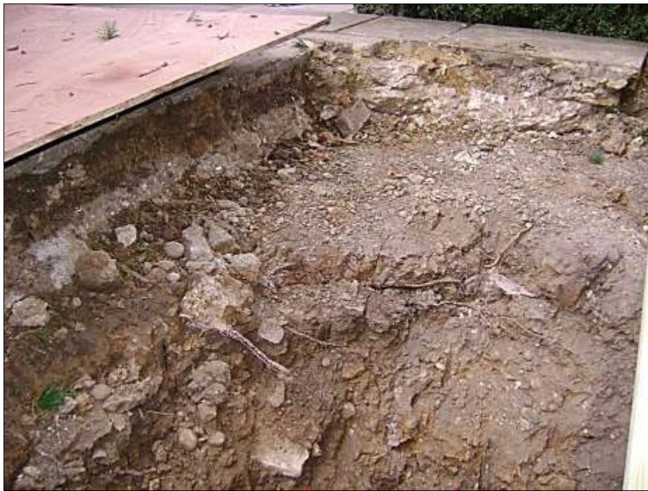
Photograph 4 – A closer view of the trial pit showing the fibrous roots and the layers of concrete, hard-core and stone debris below the surface of the stone patio.
