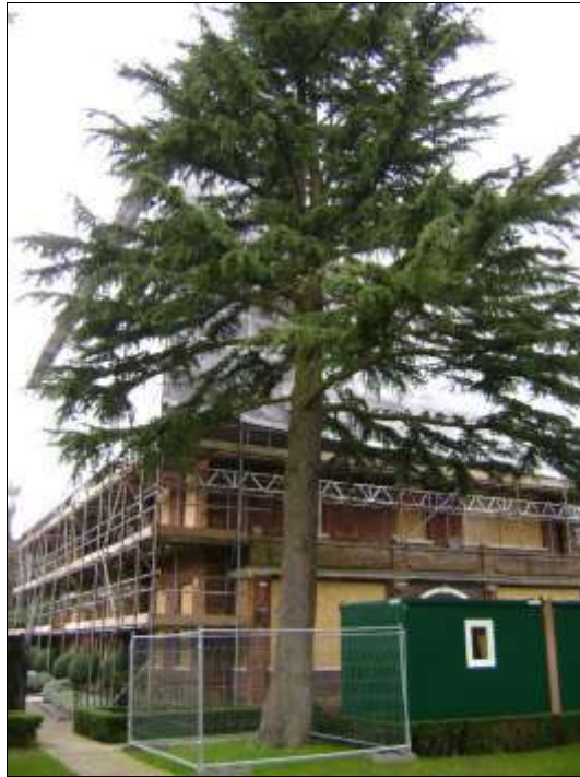
Photograph 1 – Cedar tree T1. The site cabins have been placed on the stone patio surface for the duration of the construction work. The protective fencing is a temporary measure and will be moved out to protect all the soft ground within the Root Protection Area.
