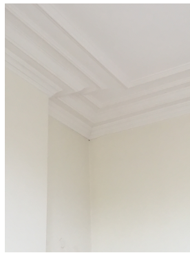
Reception Room (5101) Non original fibrous plaster cornice with combination of 3 elements; twin astragals to ceiling separating scotia to double ogee and finally minor ogee to wall
