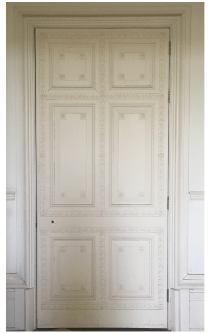
New doors to be hardwood and to match existing in materials, proportion and detail
