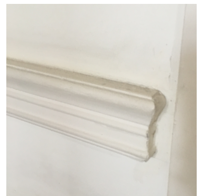
Architraves and linings to all door openings, with torus and bead quirk detail
