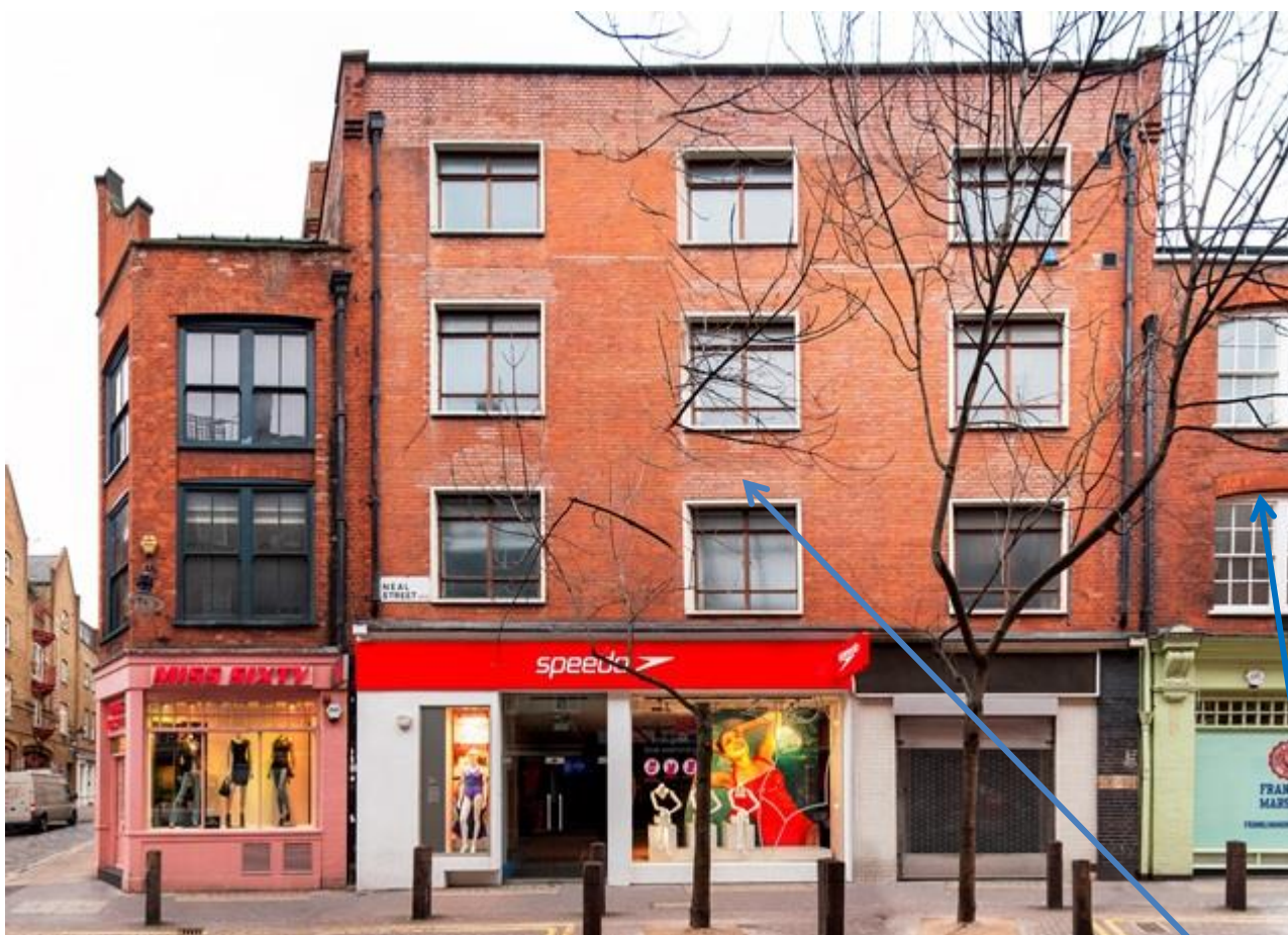
The left arrow indicate the c.1950's infill of the c.1880's brick arches on 41-45 Neal Street at 1 st & 2 nd floors.
