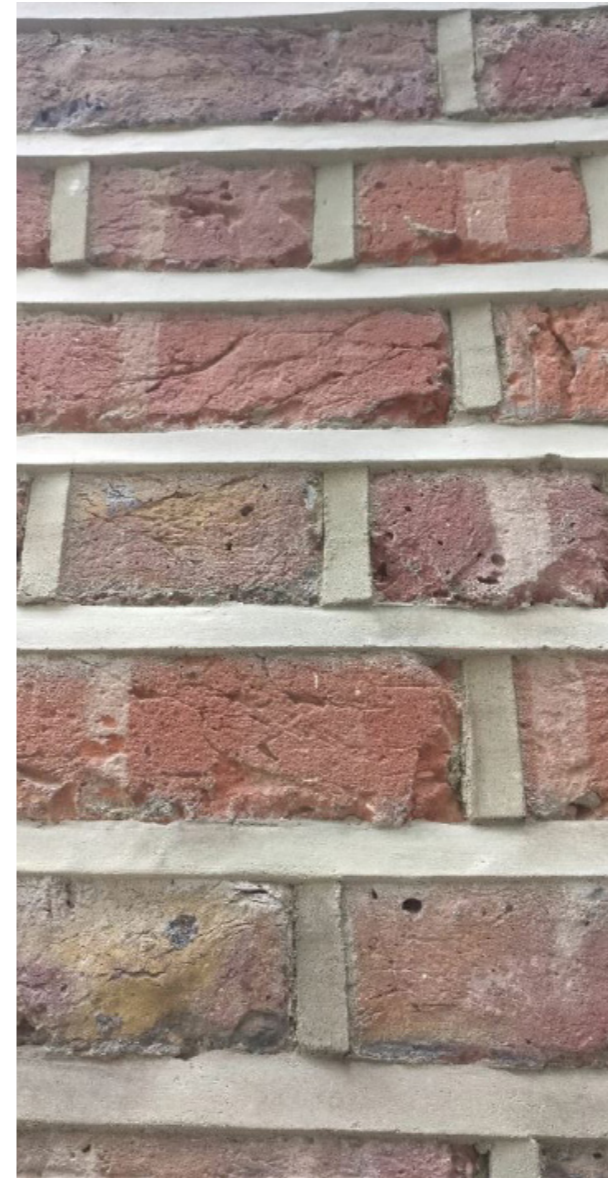
Existing wall of Wells Court, constructed with London Stock bricks using an English brick bond
