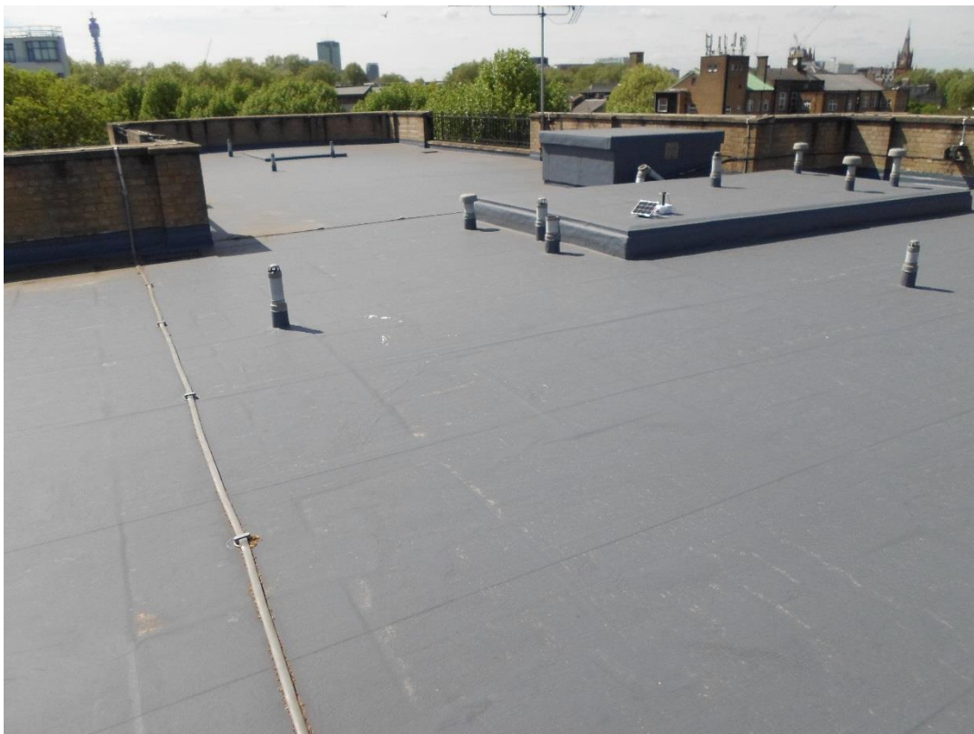
Flat roof area (looking west) – smaller area on north side of building where panels will be situated in open space avoiding protrusions. Brick wall and railing surround rooftop.
