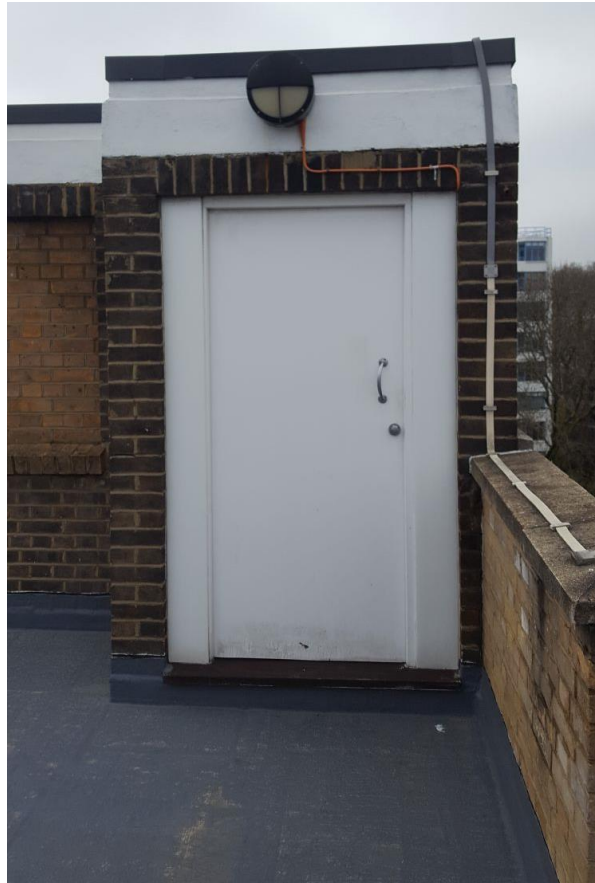
Roof access point – one flight of stairs lead down to fifth floor lift access lift
