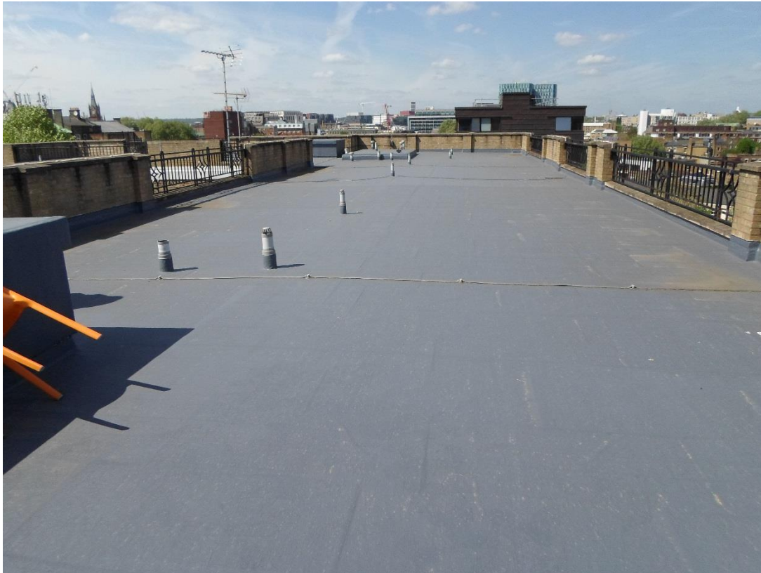
Flat roof area (looking north) – panels will be situated in open space avoiding protrusions such as small vents. Brick wall and railing surround rooftop.
