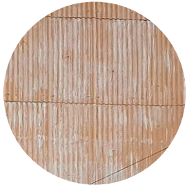
Existing Corrugated Asbestos Cladding to External Lift Shaft.
