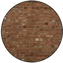
Existing Masonry Brick to Stair Core, Main Building and Single Storey Extension.
