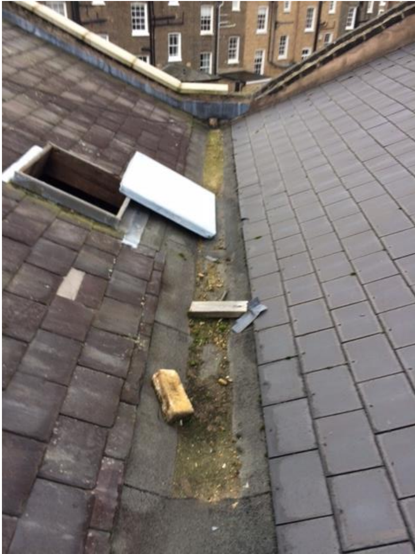
Blocked felt valley gutter
