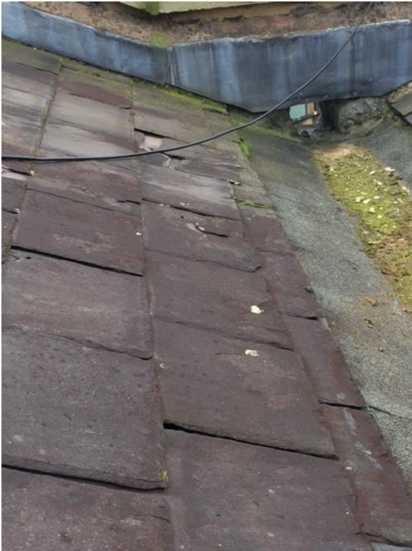
Cracked and defective slates to left hand slope
