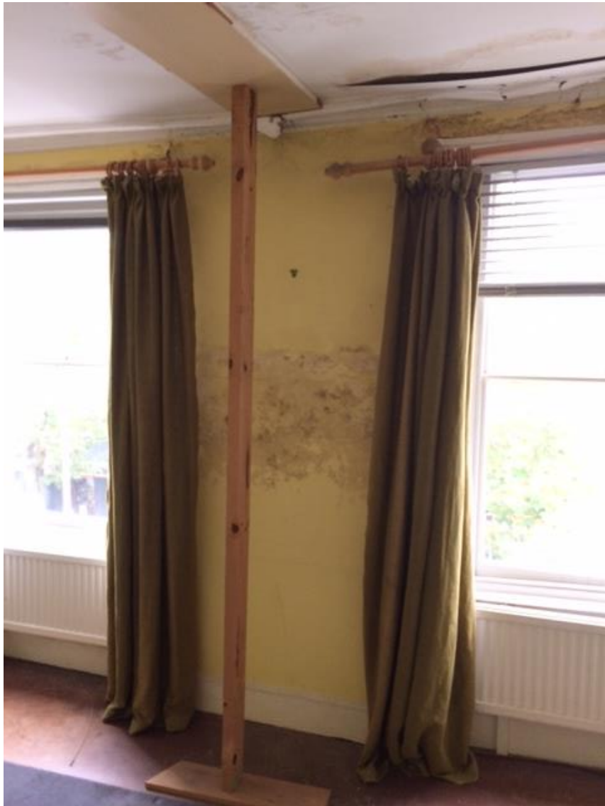
Collapsing front Bedroom ceiling and water penetration
