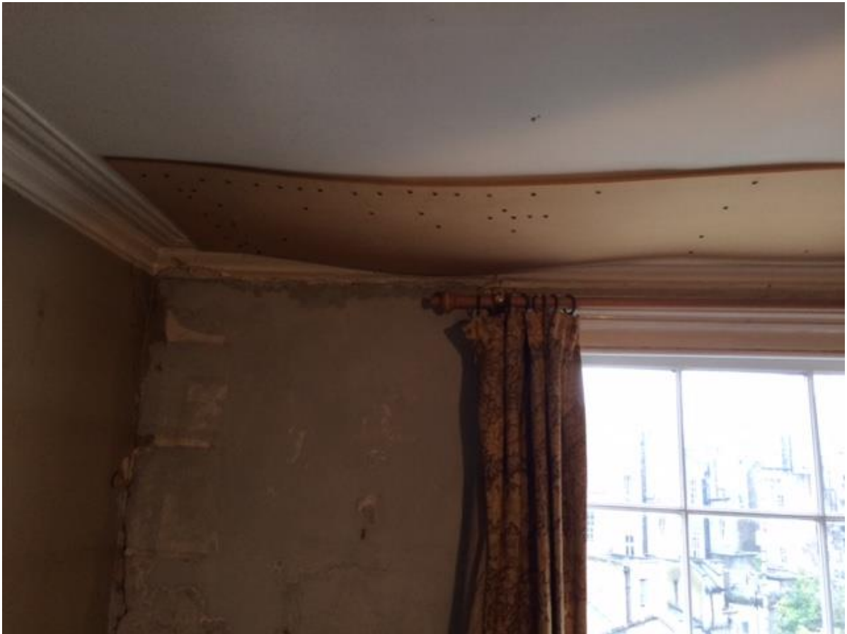
Collapsed rear Bedroom ceiling
