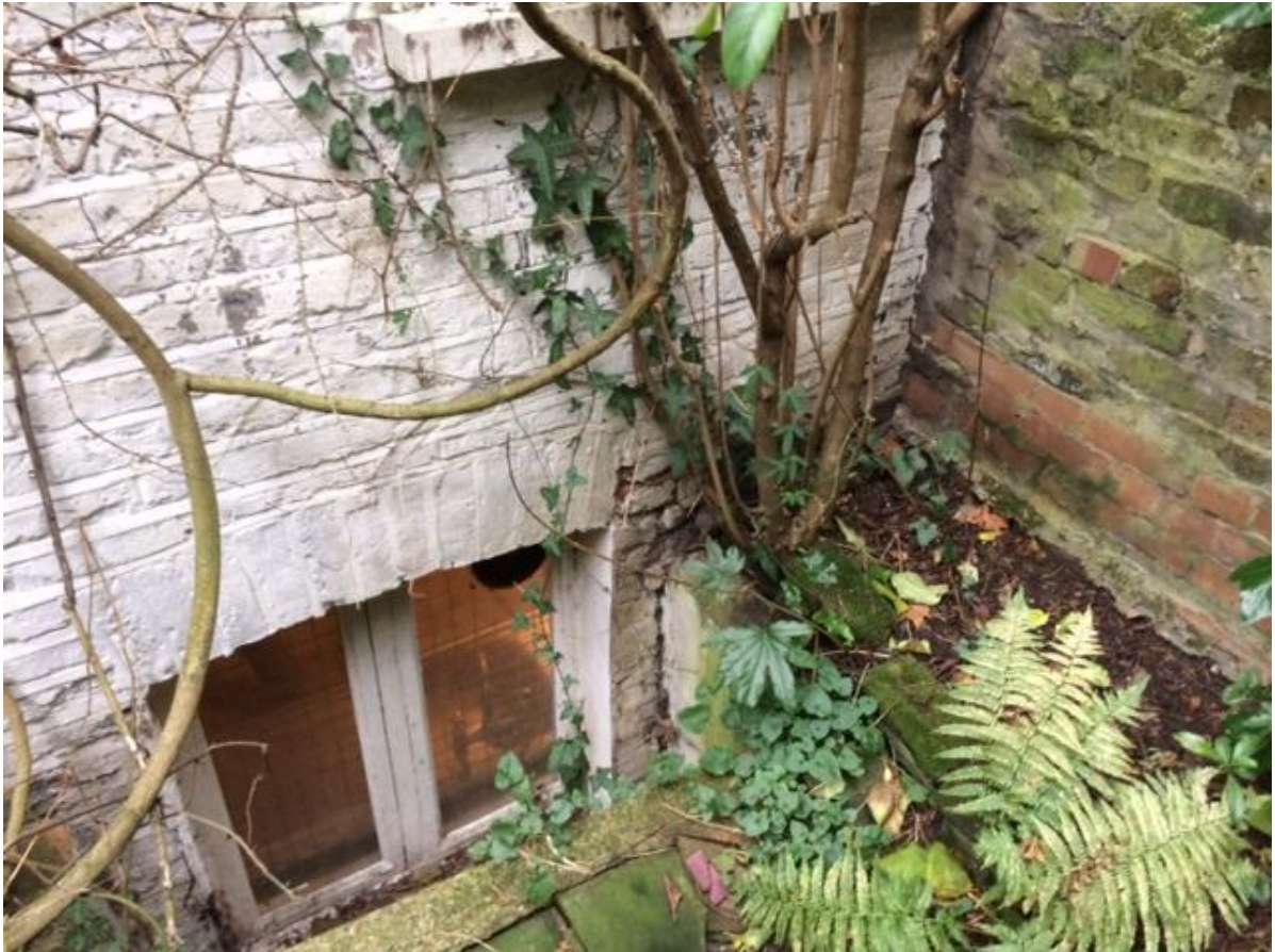
Bush/tree growing into rear addition wall
