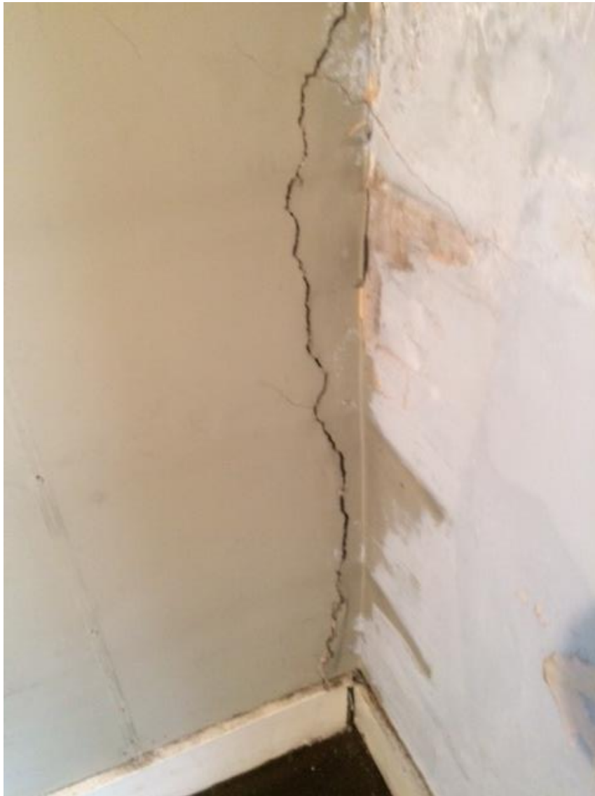
Cracking in Second Floor rear Bedroom partition
