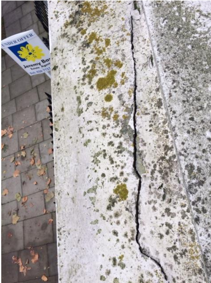
Cracking in front corbelled banded projection
