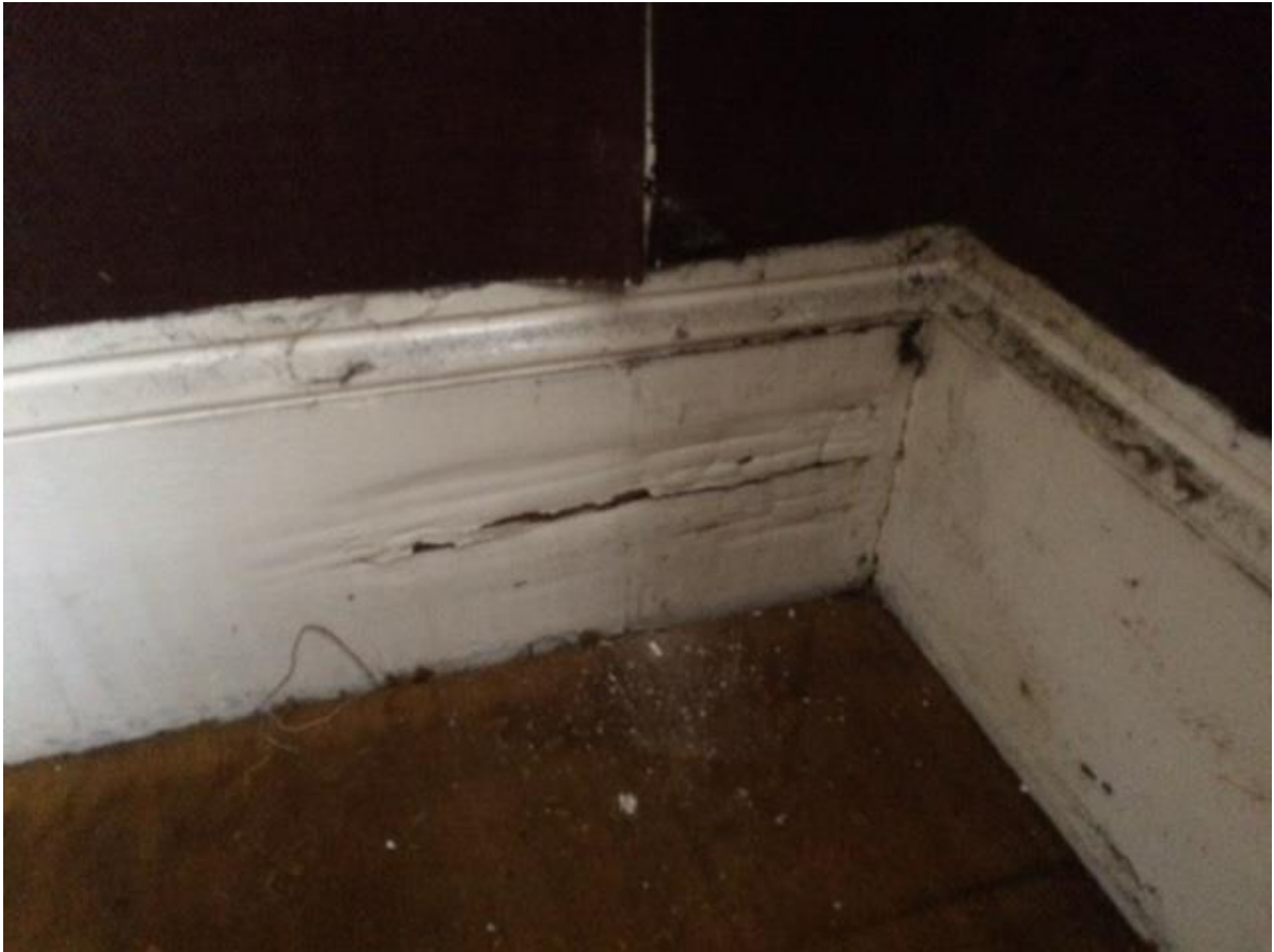
Rot infection in front Living Room skirtingboard
