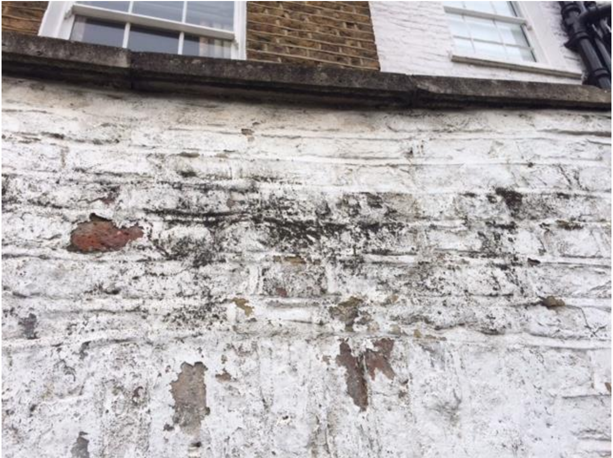
Buckled rear parapet wall
