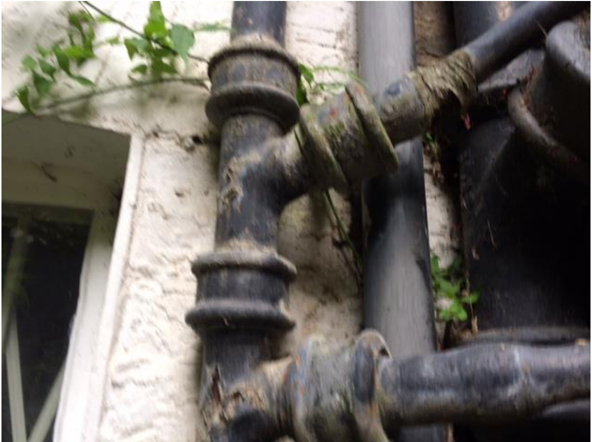
Leaking wastewater pipework
