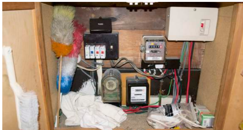
Second floor flat electricity meter
