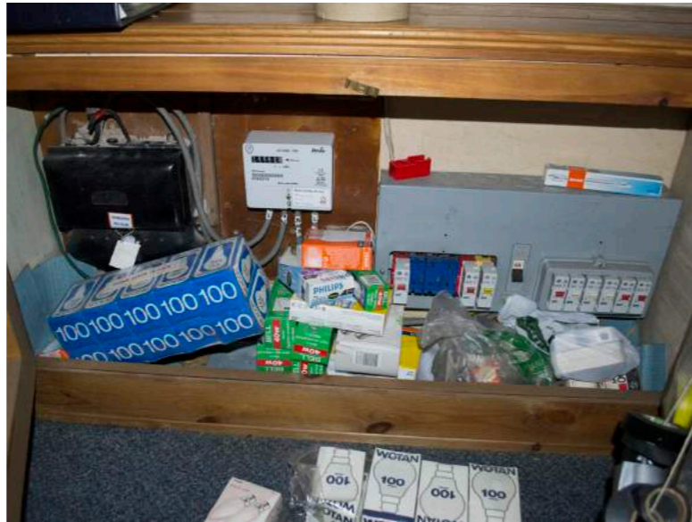
Ground/first floor flat electricity meter
