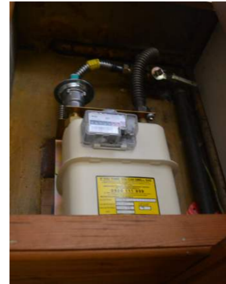
Ground floor gas meter
