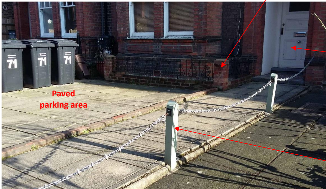
Photo 2: The parking area and path leading to the front door of No.71 slope slope towards the Goldhurst Terrace footway.
