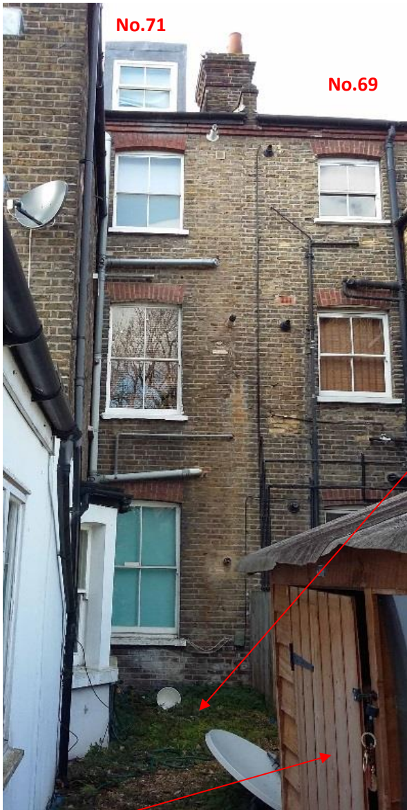
Photo 5: Rear elevation of No.71, looking north-west, showing the 'courtyard' between the rear wall and rear projection.
