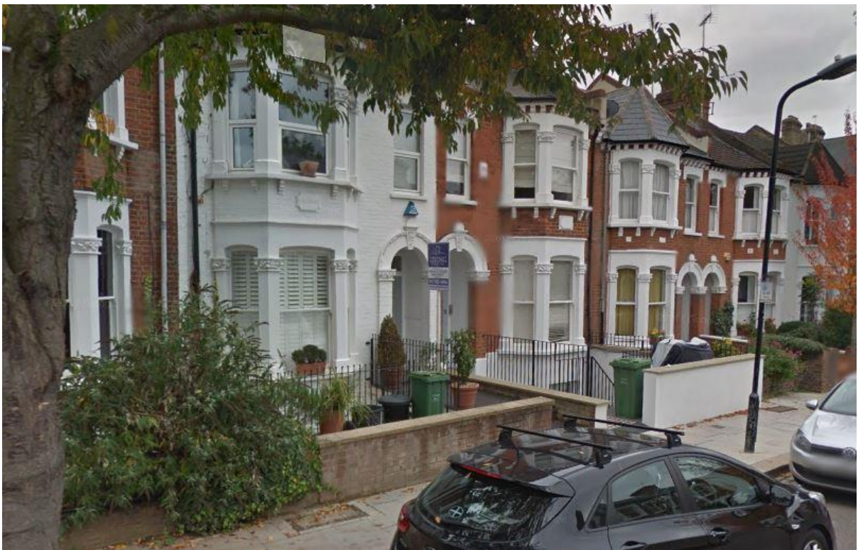
Light-well excavation, access stairs and bin storage areas completed at 21 and 23 Kylemore Road
