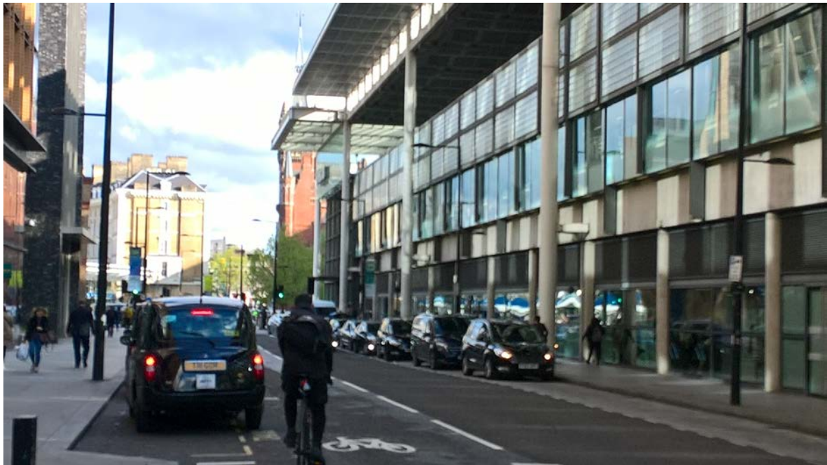
View from Pancras Road looking South onto the affected external elevation. Great Northern Hotel (Grade II) is visible in the distance.
