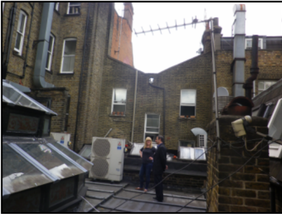
Photo 4: Existing air con units
