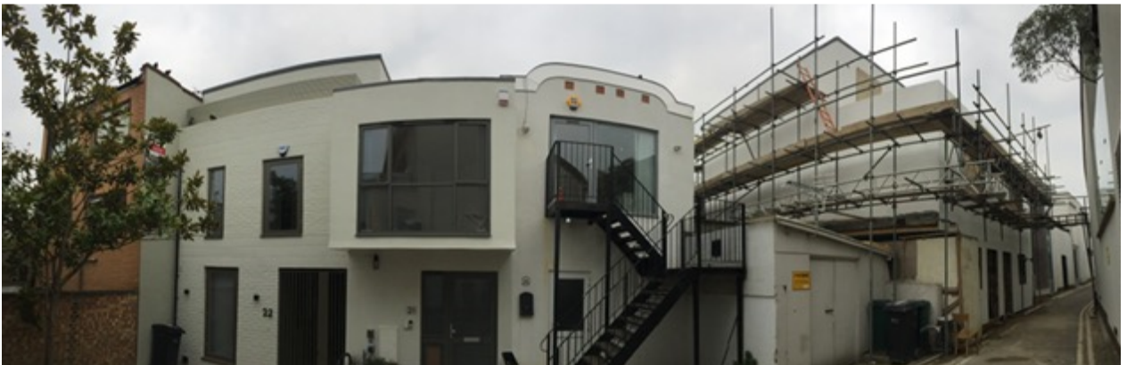
Photo 2 – View of front elevations on the east side of Rose Joan Mews
