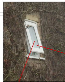
UPVC SHOWER ROOM WINDOW TO BE REPLACED WITH TIMBER WINDOW
