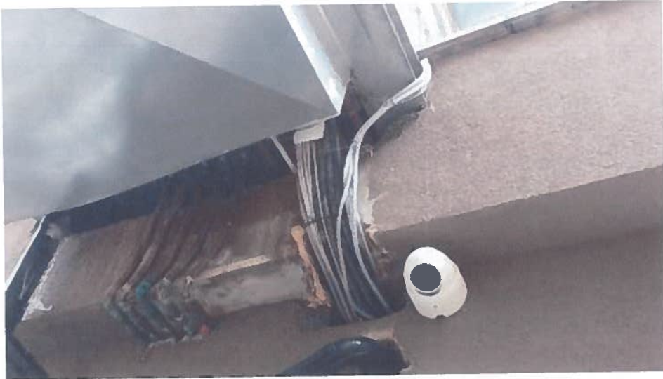
Unboxed cables, unlagged pipes, unprotected wood.
