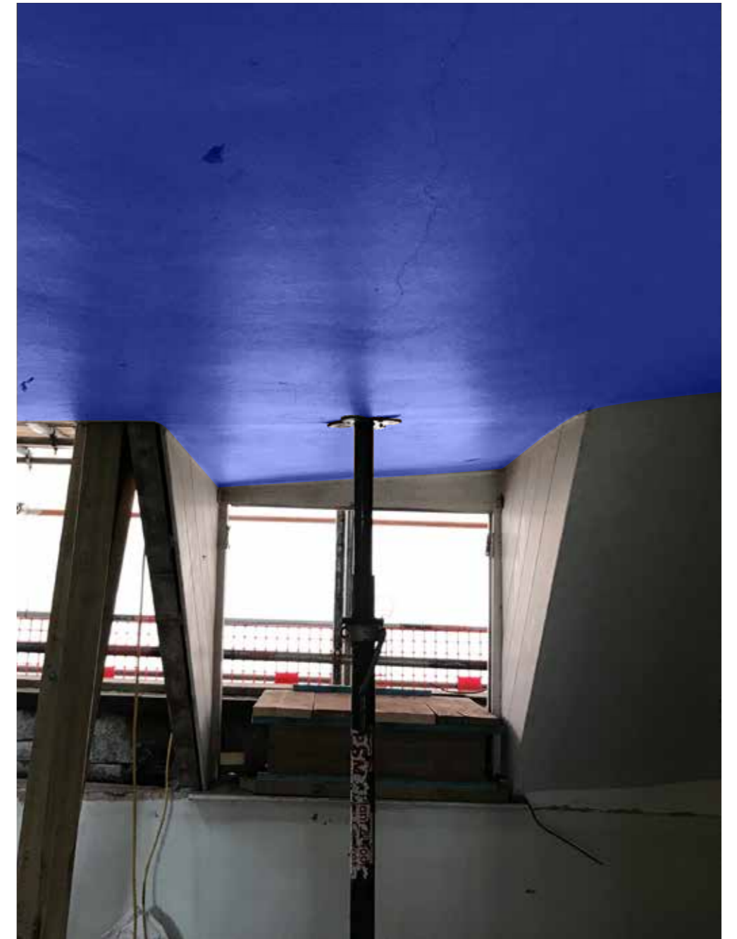
7 Denmark Street: Existing Ceiling Plasterboard to underside of lath and plaster ceiling
