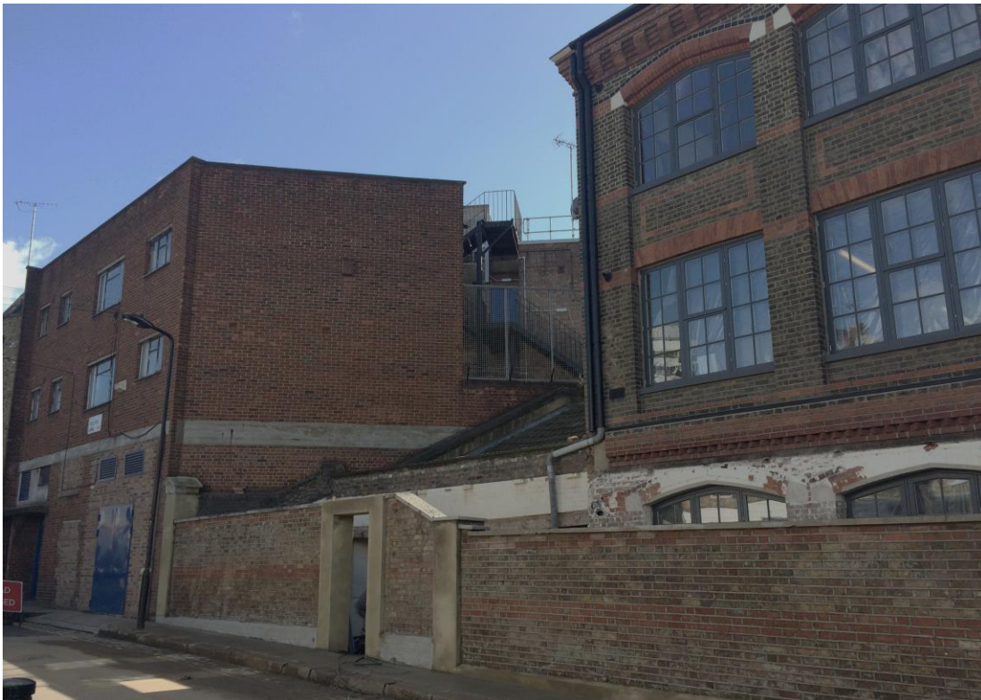
EXISTING 5 ANGLERS LANE – The void is less prominent from this angle but passers-by are still exposed to the unattractive rear of properties which are not in the Inkerman Conservation Area. This ends/starts the Conservation Area with an unsightly view
