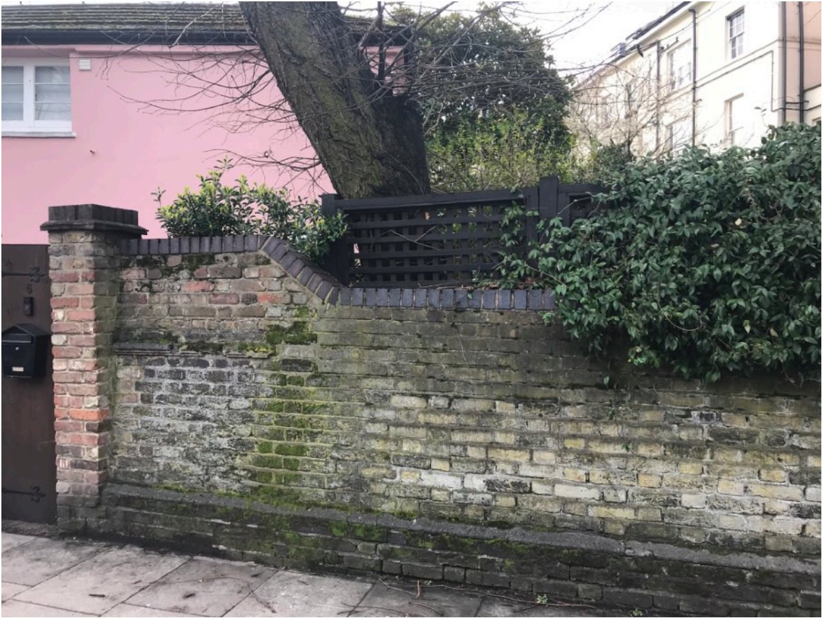
Boundary Wall showing the higher section of wall which it is proposed to match.
