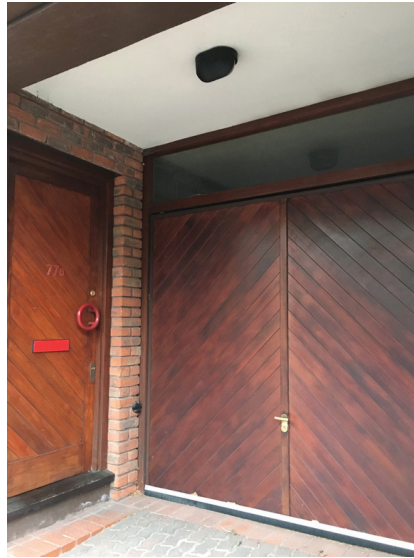
entrance and garage doors
