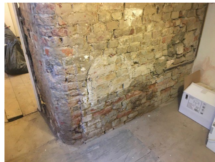
Rear of ground floor chimney breast showing poor quality brickwork, areas of non-original brick patching and cracks.
