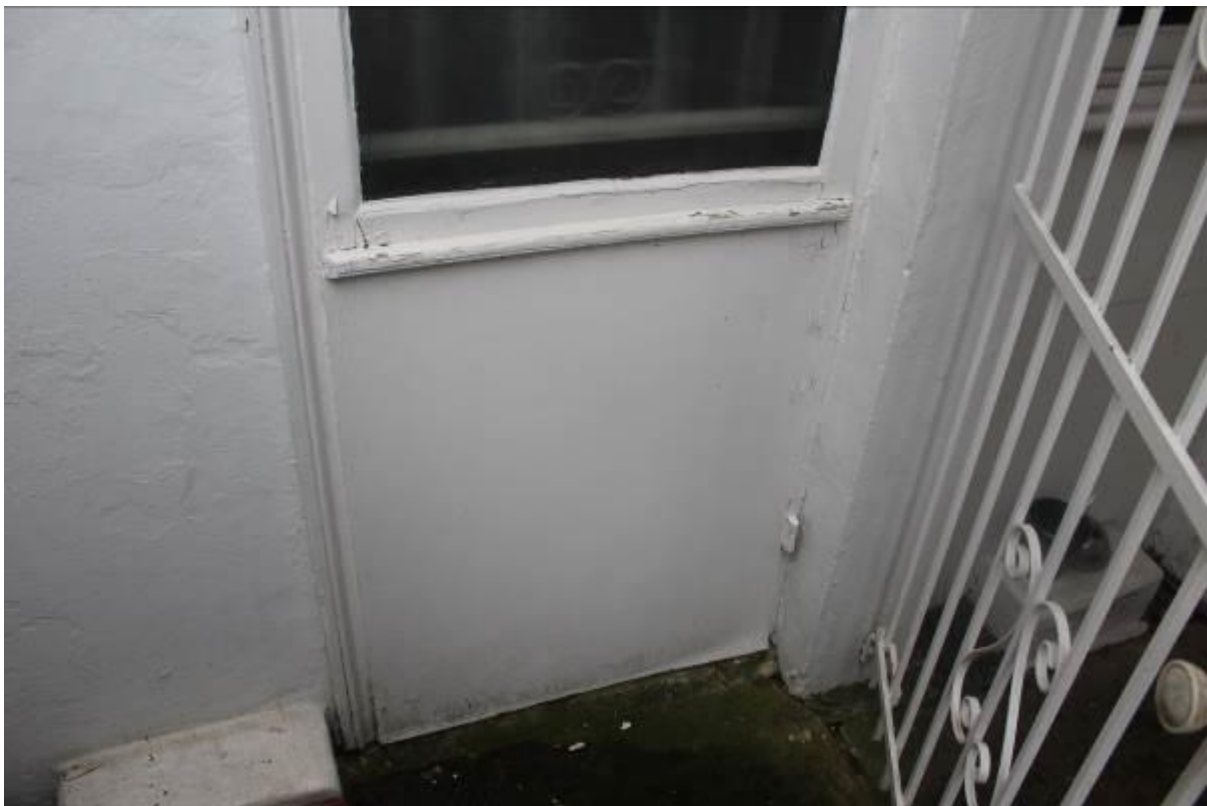
18. Rear reception room door fixed shut.
