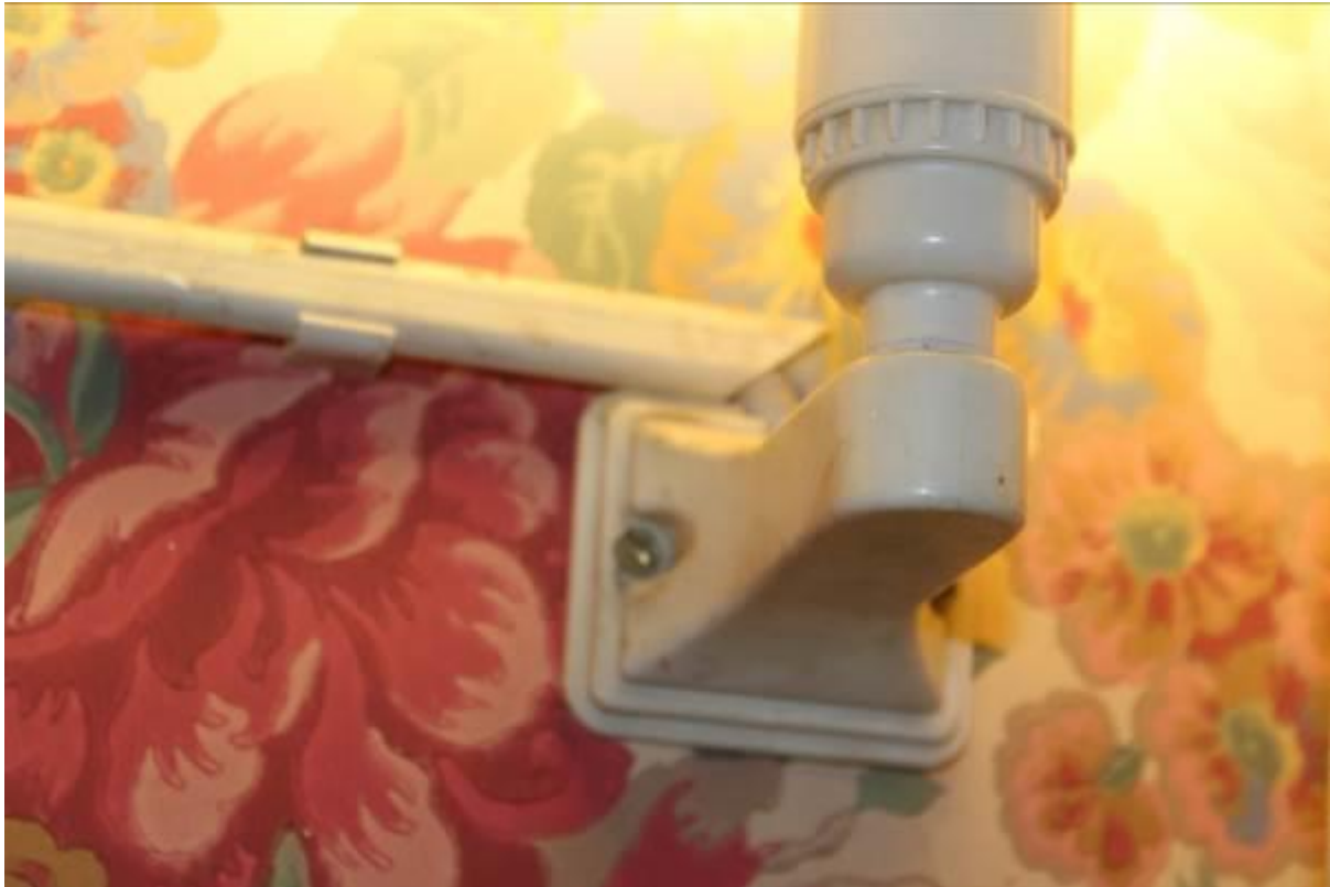
23. Poorly formed surface run conduit.
