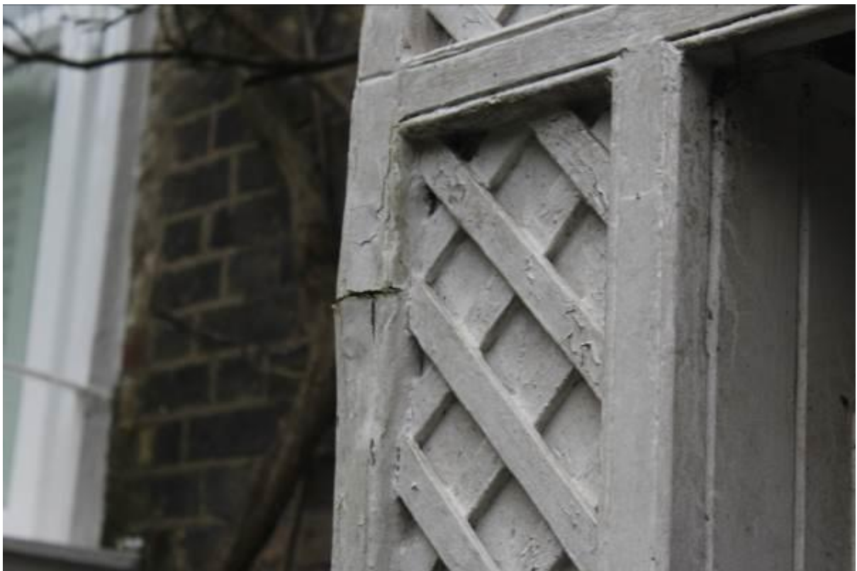
6. Window care repair required.
