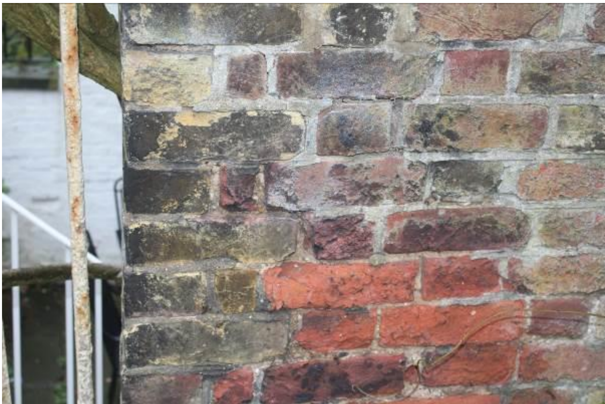
10. Some minor brick boundary repairs also required.
