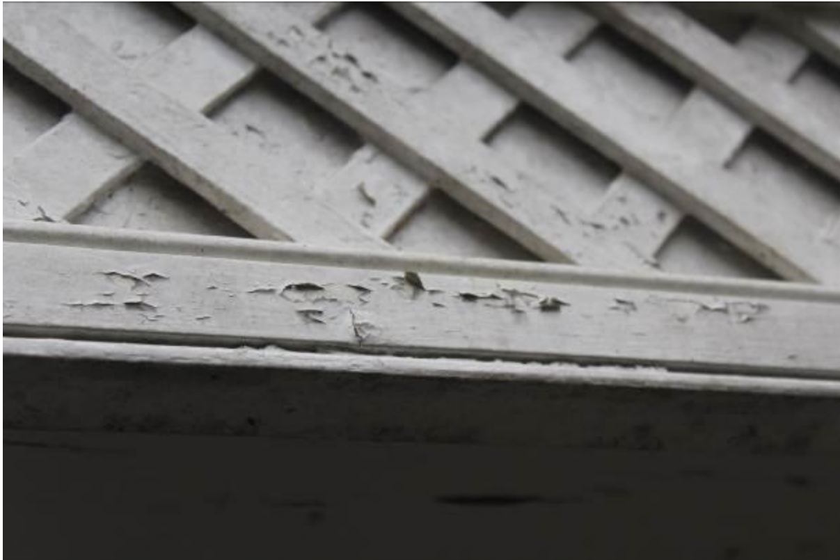
7. Paint coatings require redecoration.
