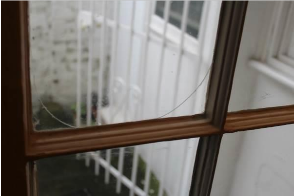
44. Replace broken glass pane.
