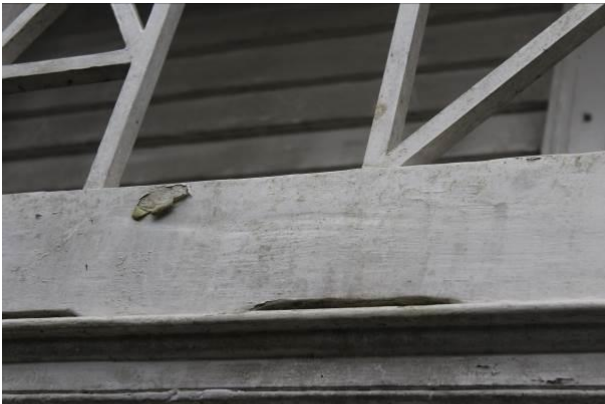
4. Timber decay evident to balcony structure.
