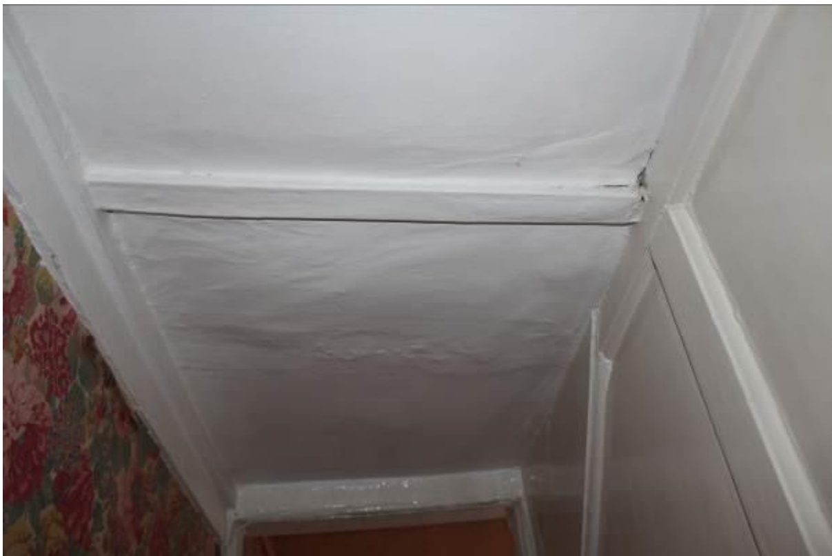
37. Overboarding recommended to first floor ceilings
