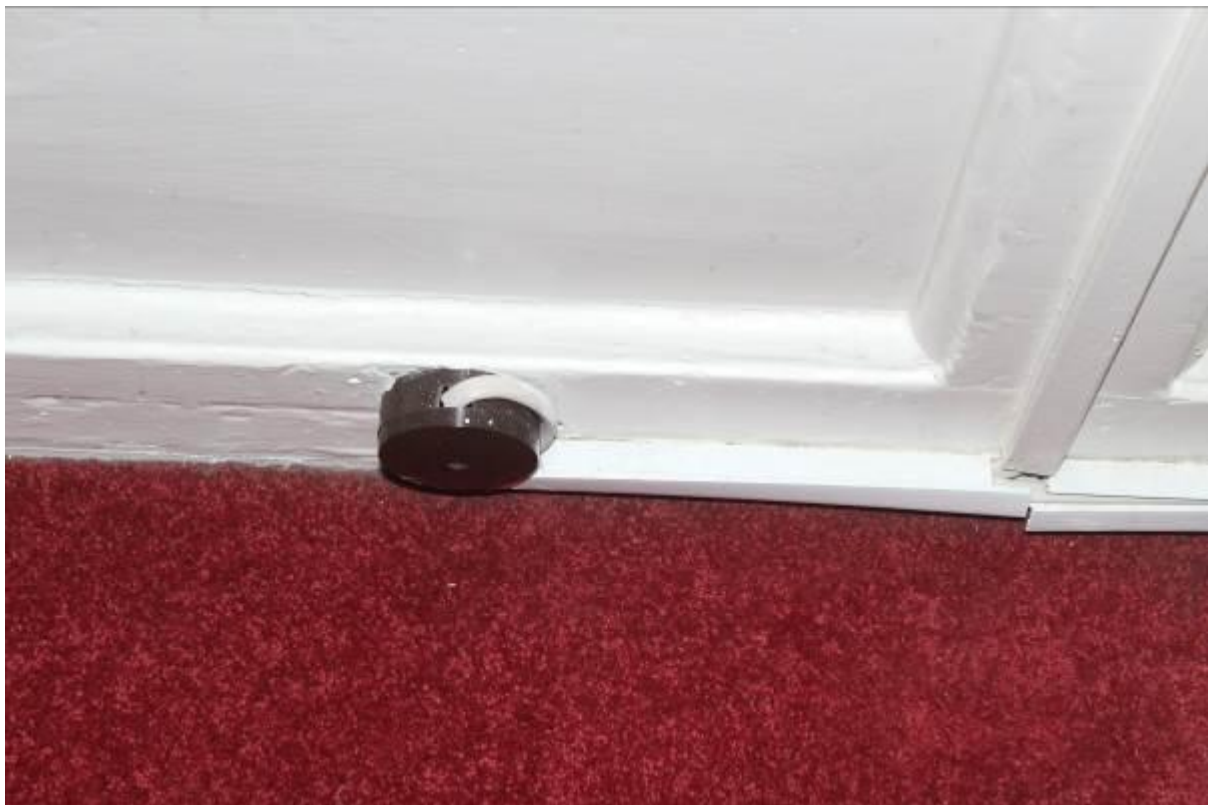
47. Poor electrical detailing.
