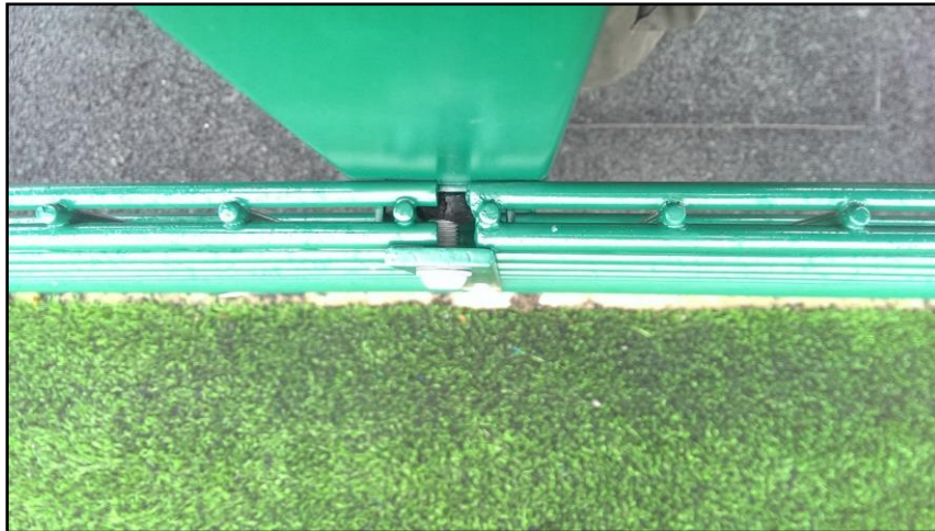
Figure 10: Image showing neoprene isolators between fence panels and post
