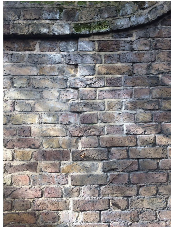
Existing cracks to wall
