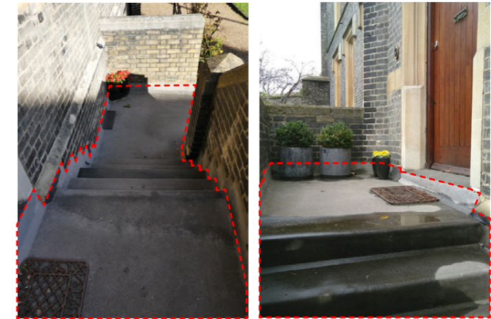
Removal of asphalt matting stair treads internally and replacement with high-quality stone stair treads.
