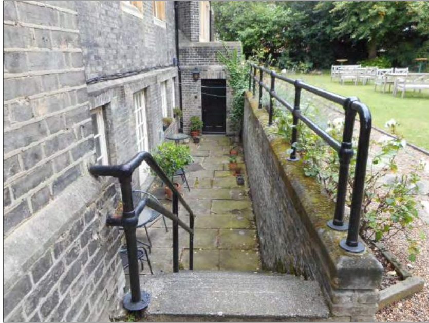
Plate 5: View of access to basement level on the western side of Nos 4 and 5 St Katharine's Precinct
