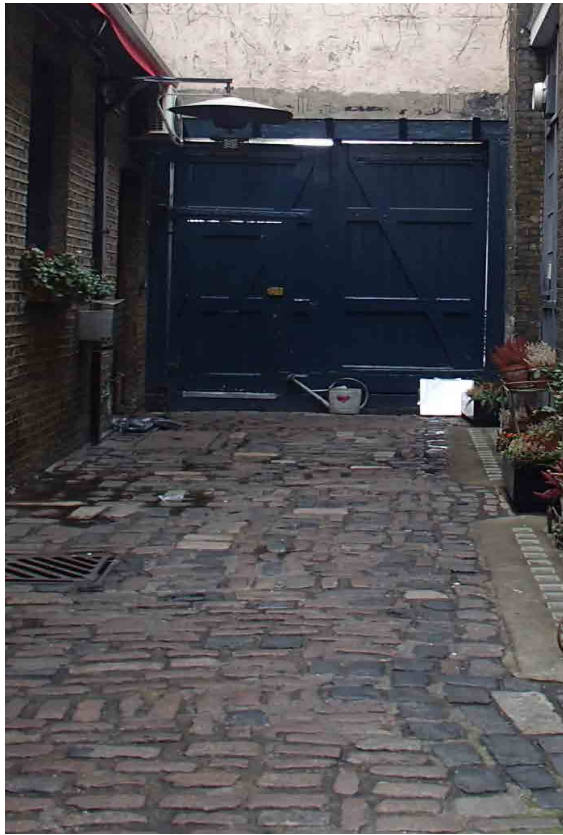
Badly re-laid granite setts, Bleeding Heart Yard
