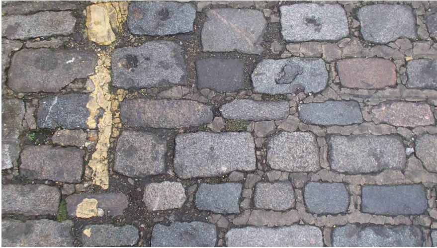
Poorly bonded granite setts, Bleeding Heart Yard
