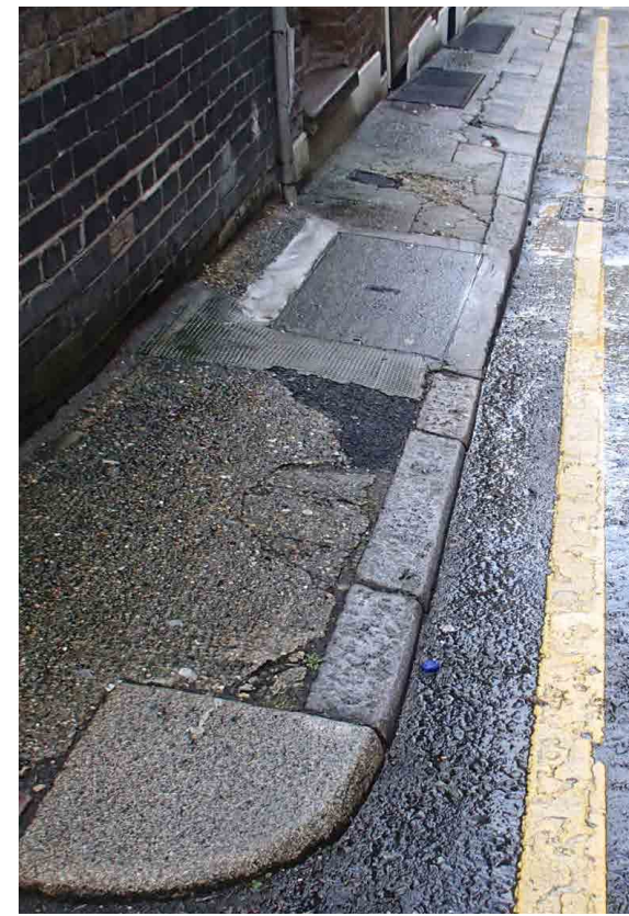
Poor-quality paving, Vine Hill
