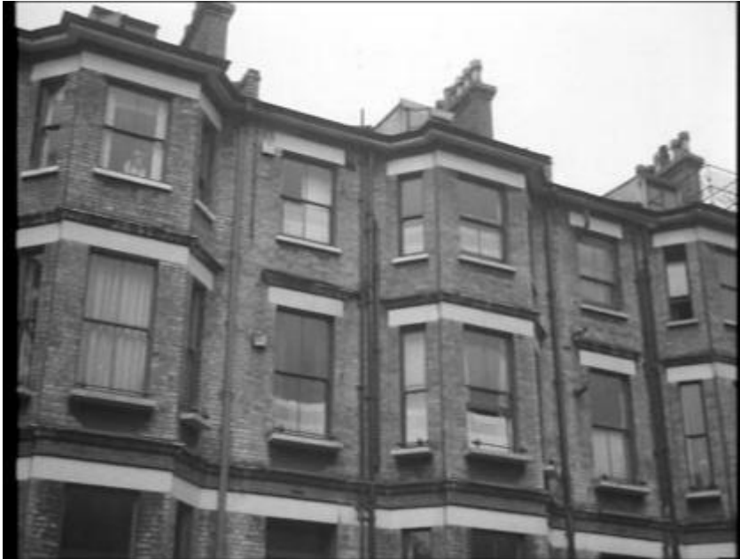
Plate 1. Photograph dating from 1957 showing railings at roof level above 2no. of the canted bays.
