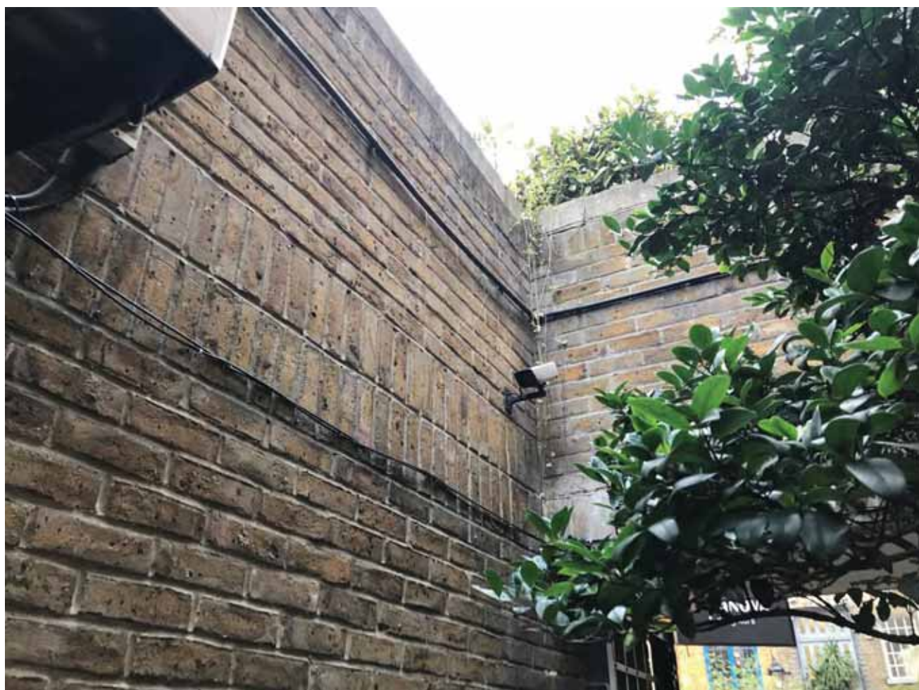
Proposed Location for Condenser Unit
