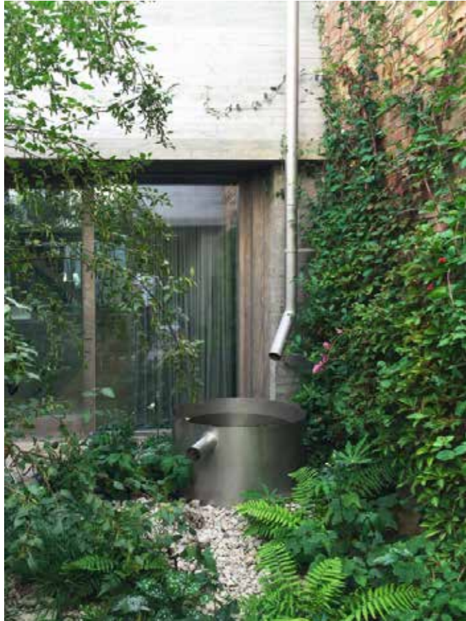
Water butts connected to RWP & SUDS
