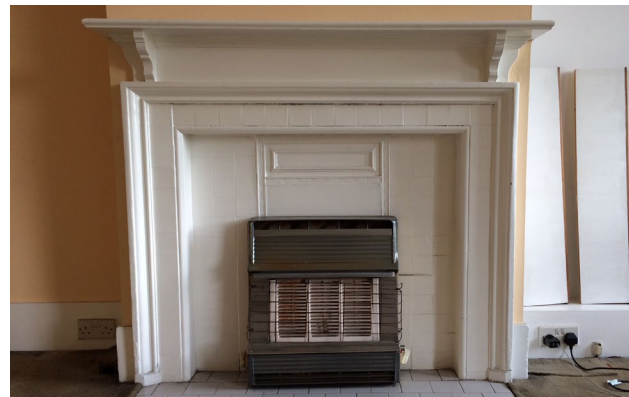
Fireplace to be replaced
