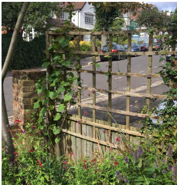
NORTHERN BOUNDARY FENCE, TO BE REPLACED WITH CLOSEBOARD FENCE TO TOP OF PILLAR WITH TRELIS ON TOP.
