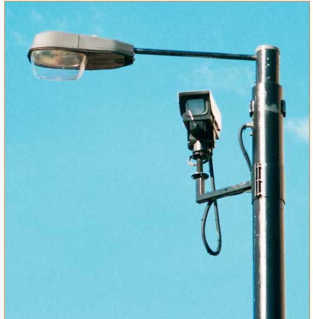
Combined CCTV and lighting column
