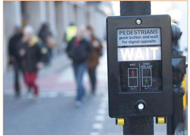
Traffic signal box with rotating 'tactile' cone (not visible)
