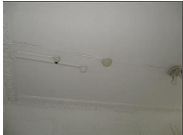
Two fire alarm systems in the flats.
