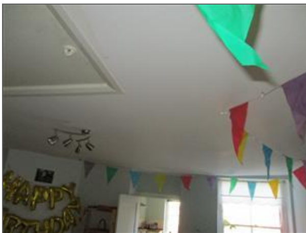
No AFD in access rooms.
