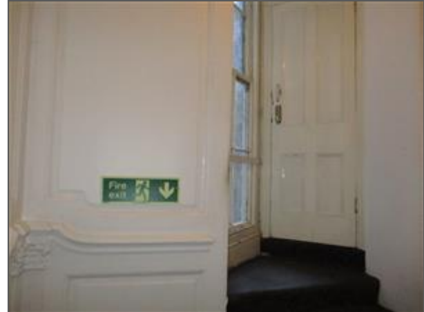
The toilet door off of the staircase does not need to be upgraded to a fire door.
