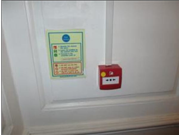
Fire action notice adjacent to the break glass call point.
