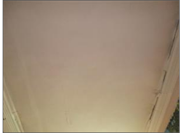
No AFD in access rooms.
