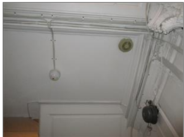
Redundant fire alarm should be removed.
