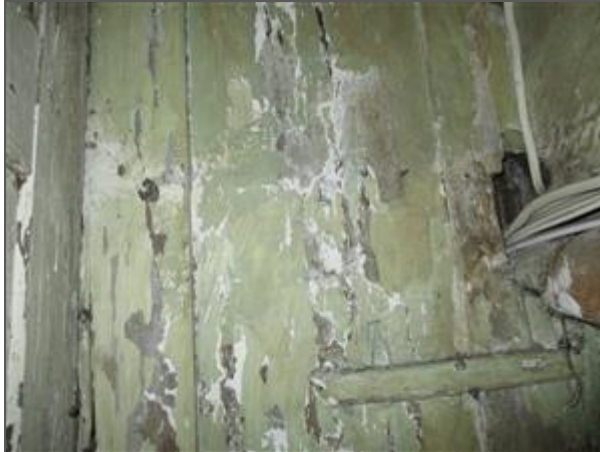
The unprotected wood in the cupboards adjacent to the basement means of escape to the front of the building that cannot be encapsulated should be treated with a fire retardant paint or varnish to provide 30 minutes fire resistance.
