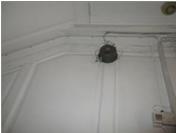
Redundant fire alarm should be removed.
