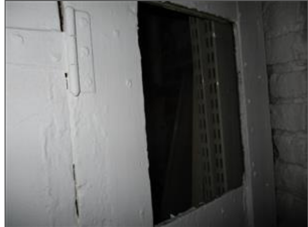
The openings in the basement office walls adjacent to the basement means of escape to the front of the building by ducting or building services should be fire stopped using approved materials installed by a competent contractor to provide a minimum of 30 minutes fire resistance.
