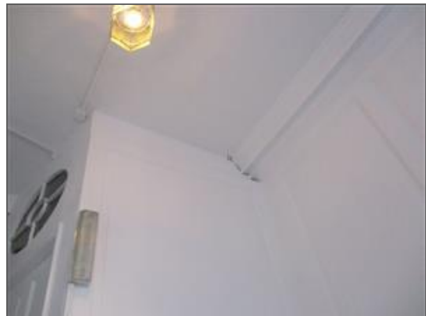
On the staircase by Flat 2 the wall needs to be fire stopped to provide a minimum of 30 minutes fire resistance.
