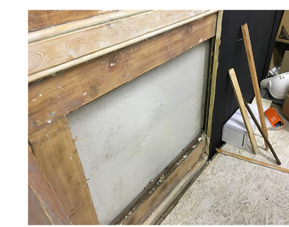
ASBESTOS PANELS OBSERVED BEHIND TIMBER WALL.
