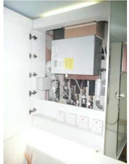
Bathroom - Detail showing the access panel for the plumbing and electrical services.
