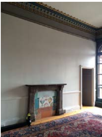
Room 2 - East elevation showing the original stone fire surround and passage to room 3.
