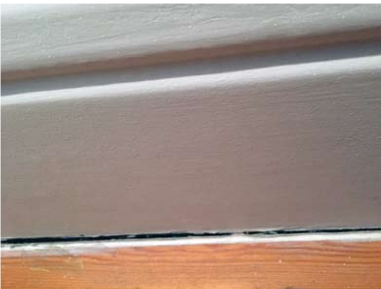
Detail showing the gaps and mastic between the floor and the skirting
