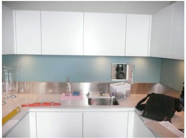
Room 3 - Kitchen detail showing the access port to the wall cavity housing building services.
