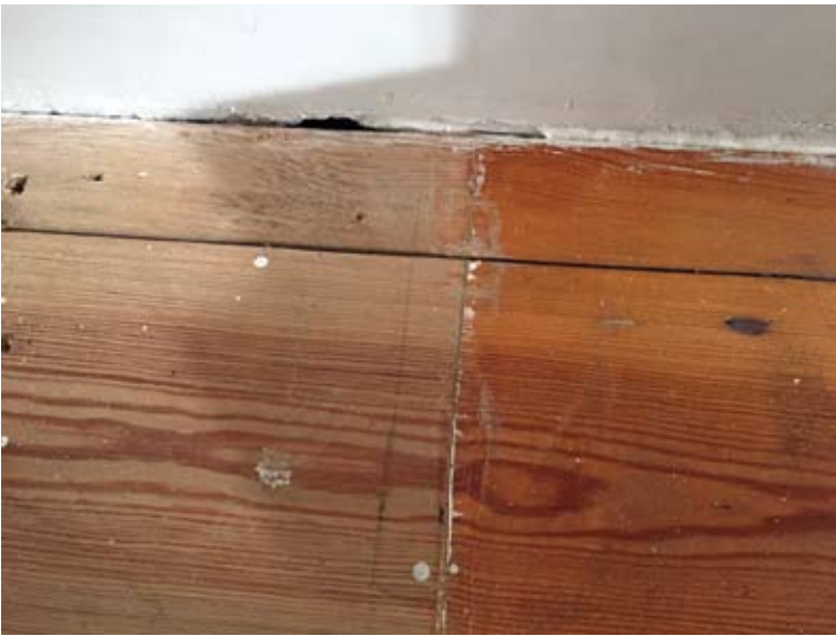
Detail showing the bare floor finish exposed by the removal of a piece of new fitted furniture, contrasted with the adjacent polyurethane varnish finish.
