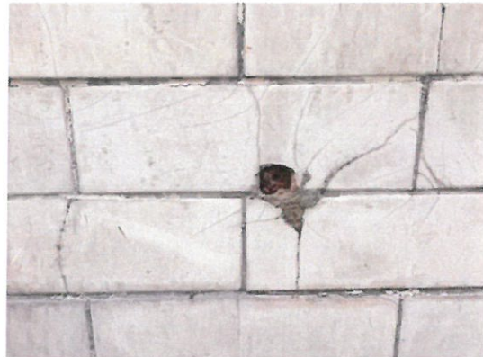
Impact damage, previous wall fixing damage
