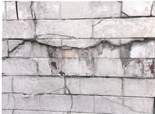
Exterior wall, severe movement and moisture ingress
