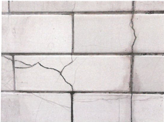
Movement cracks causing surface cracks / fissure
