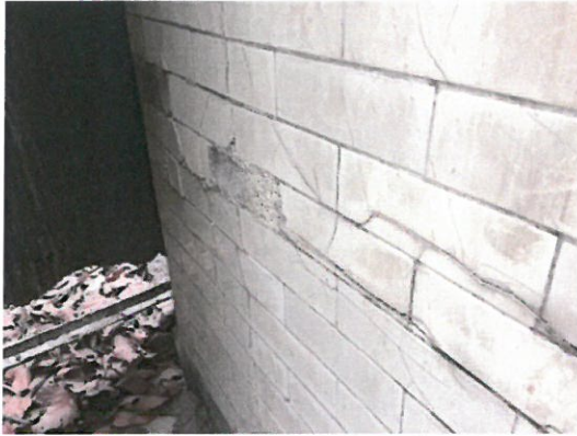
Structural failure, horizontal crack
