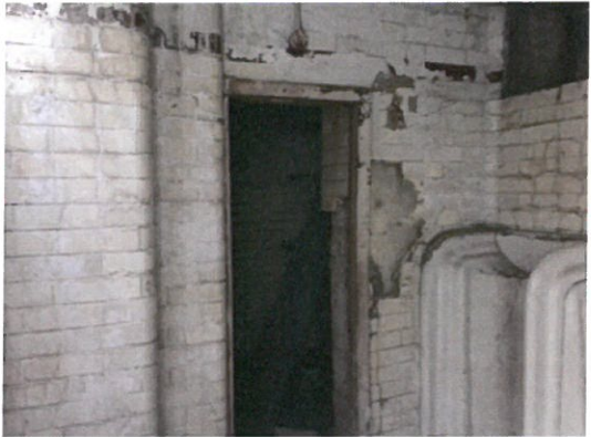
Paint in tiles surface, numerous missing sections
