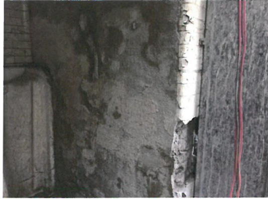
Large rendered section, missing tiles
