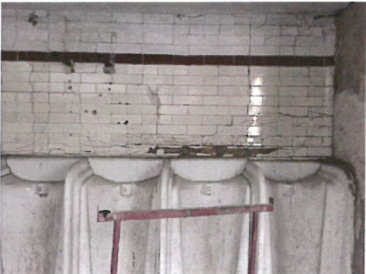
Delaminated tiles above urinals
