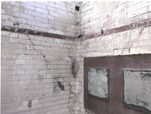
Severe structural crack, wall paint on tiles
