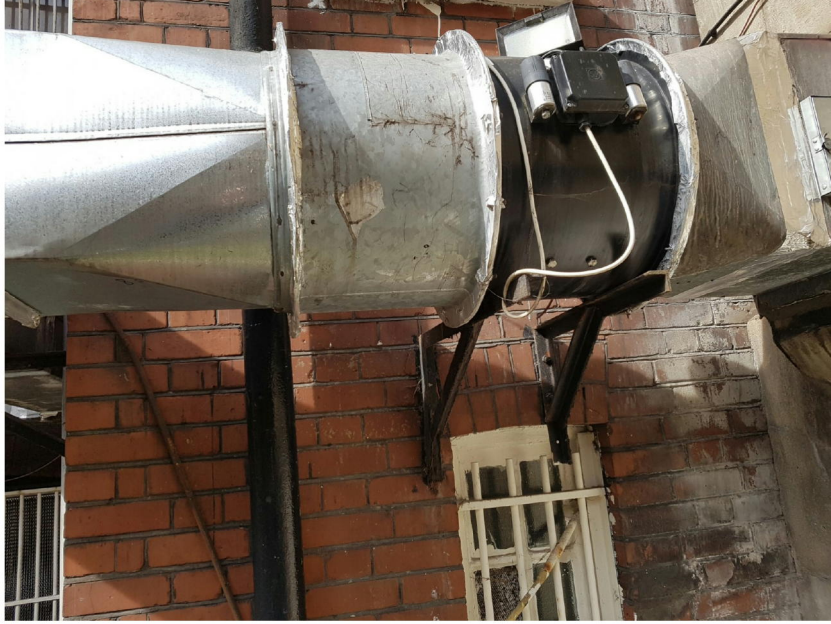
Extract motor at Humaira Restaurant 110 Judd Street, motor is mounted on outside of building and stood away from the wall to limit noise and vibration.
