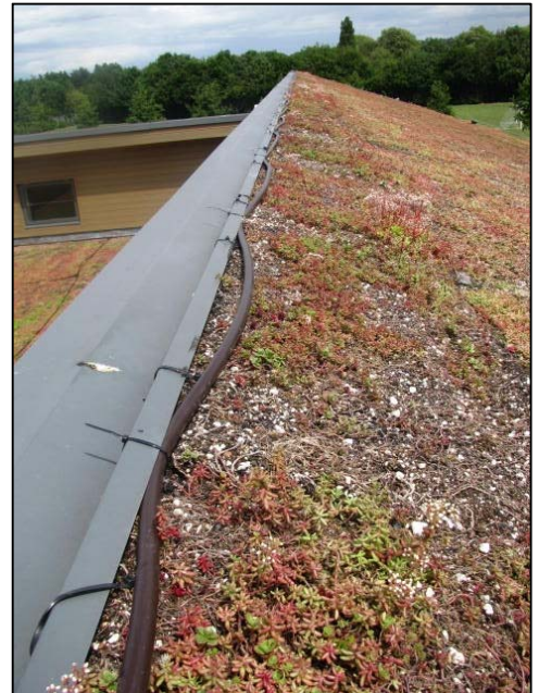
Sedum blanket being applied to a steep sloped roof, fitted with both retention strips and drip line irrigation.
