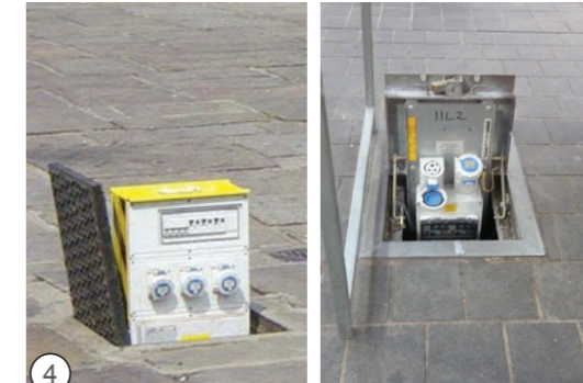
4 Power and data pop-up units
