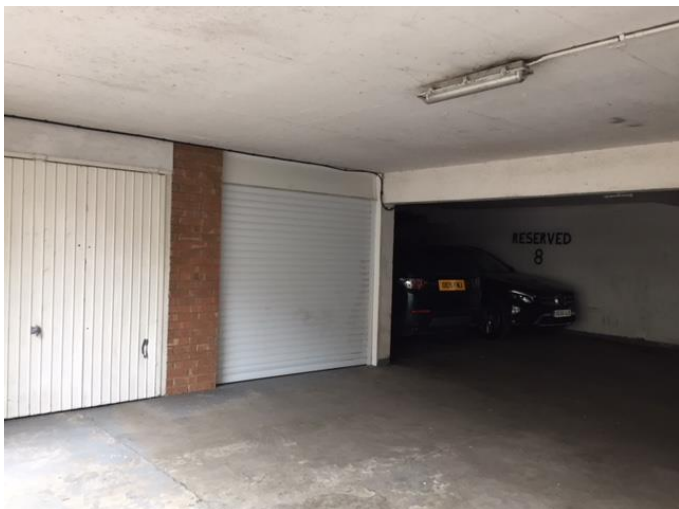
Photo 8 (above): Existing garages and parking spaces at basement level beneath front forecourt
