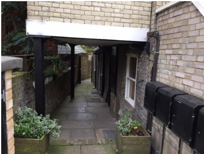
Photo 6 (above): Existing side windows and entrance door to lower ground floor flat 13a Crossfield Road
