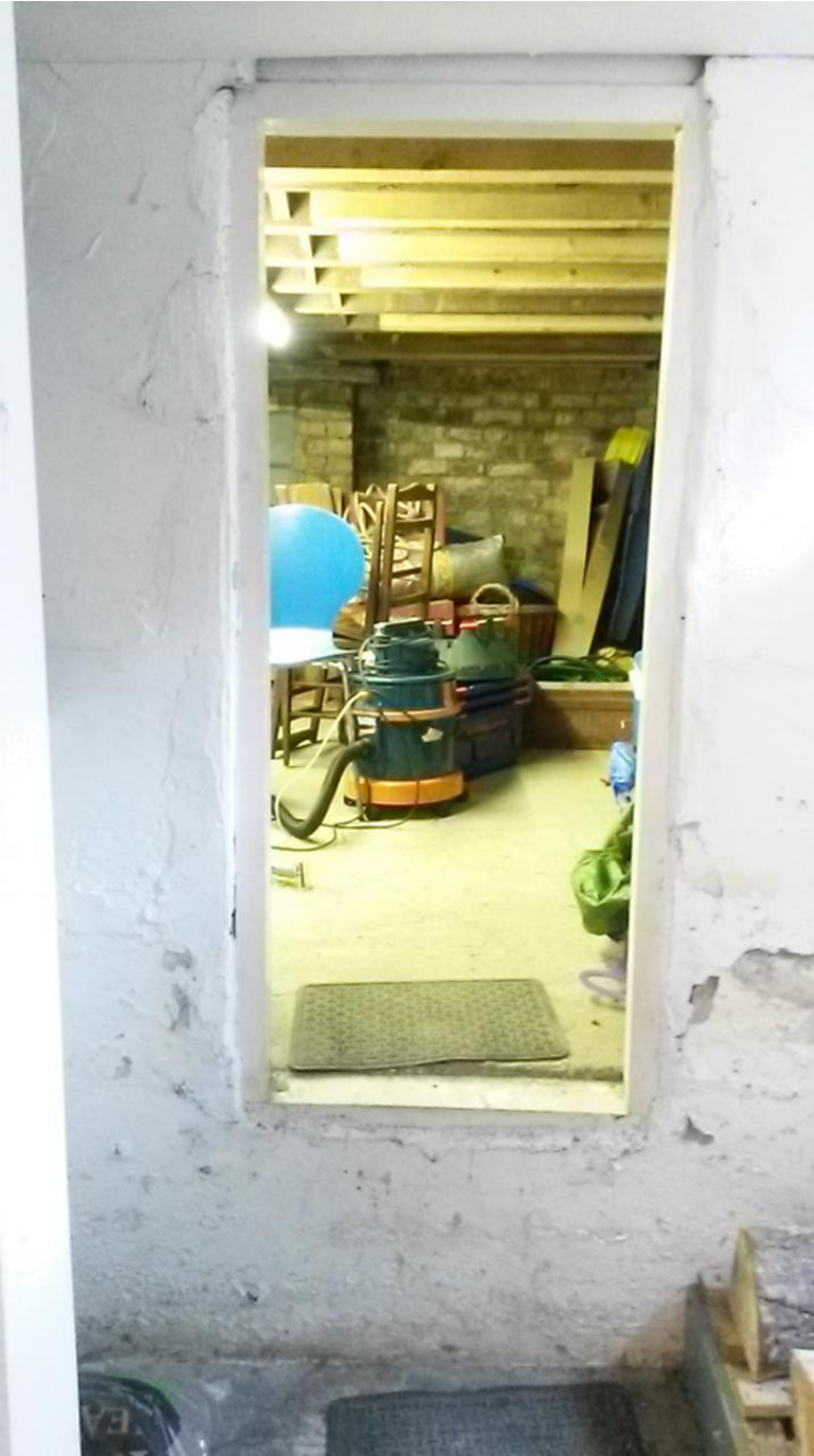
Photo 4 (above): Existing crawl space beneath front ground floor living room of 56 Croftdown Road
