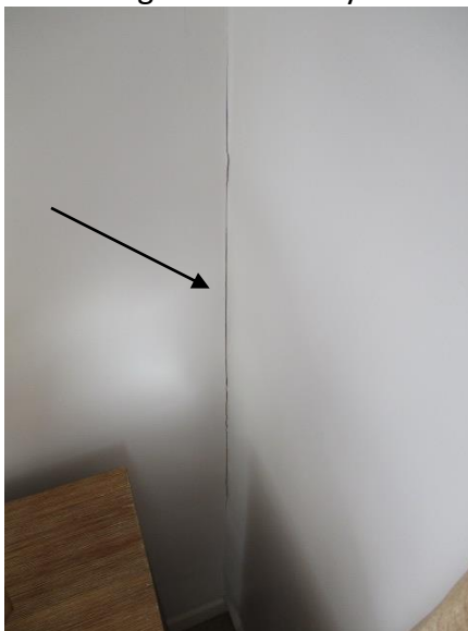
Cracking in flat 3 front bedroom
