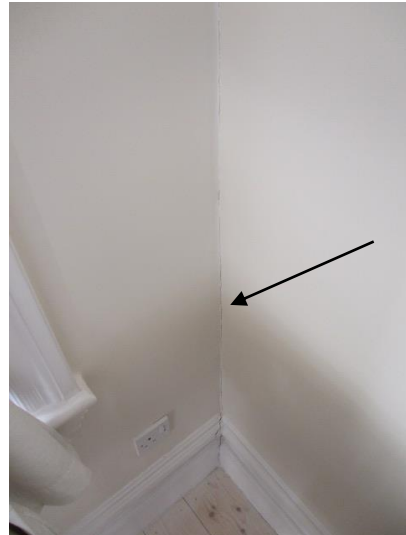
Cracking in flat 3 lounge
