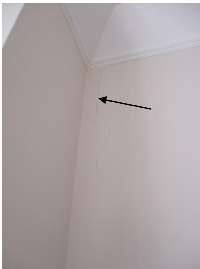
Cracking in flat 1 front bedroom
