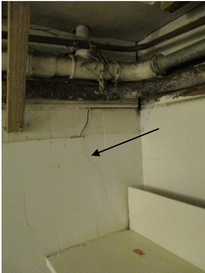
Cracking in flat 1 utility room
