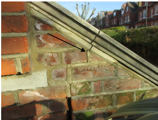
Cracking to left hand side of steps
