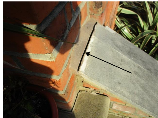
Cracking to right hand side of steps
