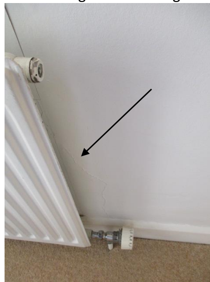
Cracking in flat 3 front bedroom
