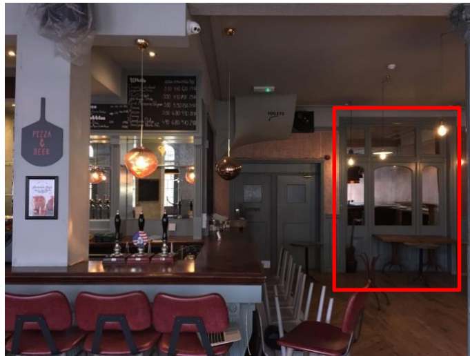
Photograph 5 – showing the opening to be blocked up between the existing kitchen and bar area.
