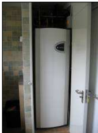
Figure 7: Domestic Scale Heat Pump
